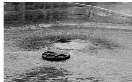
SSOs can occur at numerous locations in the sewer system, including at manholes.
