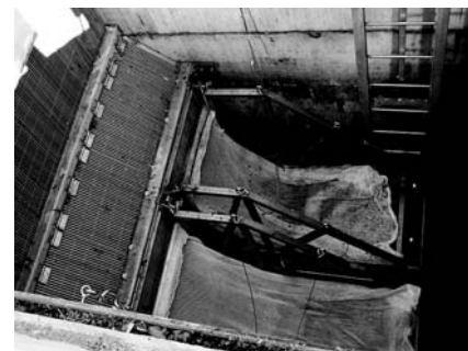
In 1999, North Bergen Municipal Utilities installed numerous mechanical screen bars and netting systems to control solids and floatables in CSOs. The facilities cost $3.3 million and annually cost $57,373 to operate and maintain (2002 dollars).
