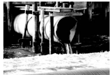
Typical CSO outfall discharge following a storm.
