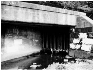
A CSO outfall in Wilmington, Delaware.
