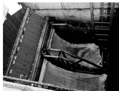
In-system netting can provide floatables control at strategic locations in the sewer system.
